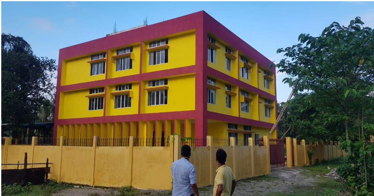
Construction of District Library Building including Equipment etc at Bijni Sub-Division under One Time Special Grant for 2017-18(On-going work)
