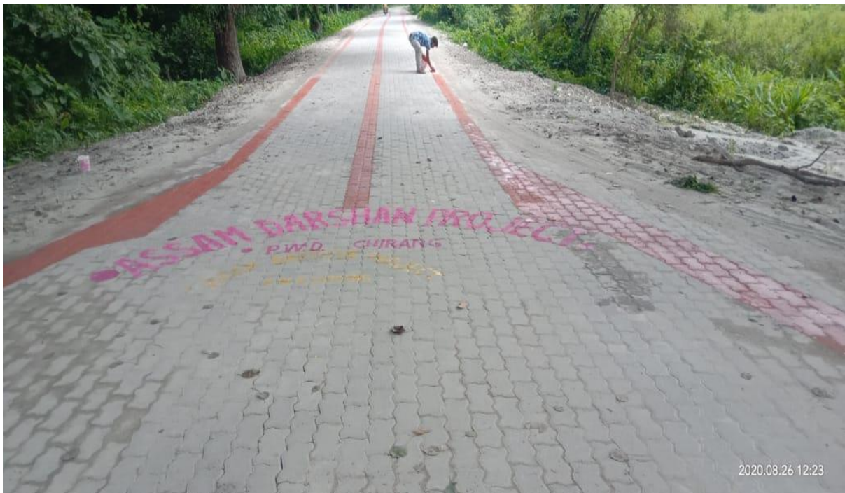
Upgradation of approach road to Jyoti Ashram Roumari from Chapaguri Amteka road under Assam Darshan in Chirang District for the year 2019-20(Completed)
