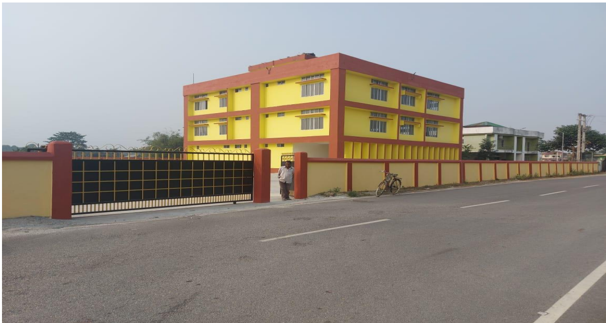
Construction of District Library Building including Equipments etc at Kajalgaon Sub-Division under One Time Special Grant for 2017-18(On-going work)
